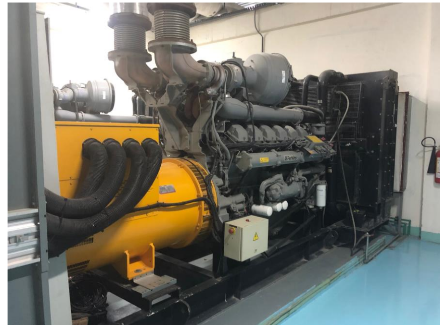
Diesel generator Source: BSW
